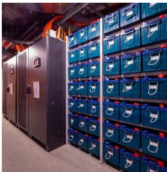
New UPS units and batteries
