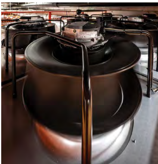
High-efficiency computer room cooling fans
